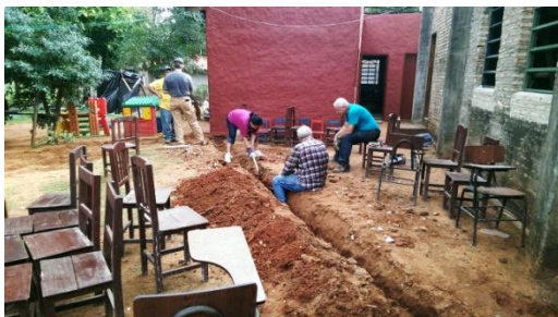
Digging a trench for the electrical conduit for the church building at Barrio Parque.
