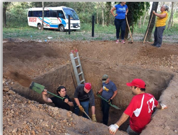
Work on the septic tank for the toilets at the Marin site.
